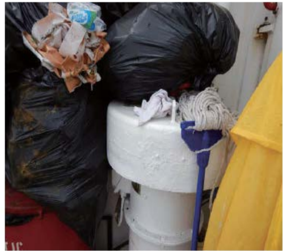
Ventilator is obstructed by garbage
