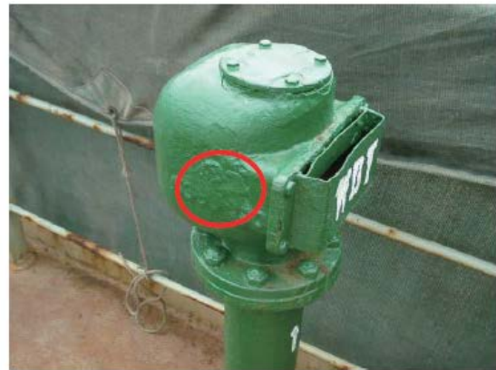
Inappropriate temporary repaired by putty
