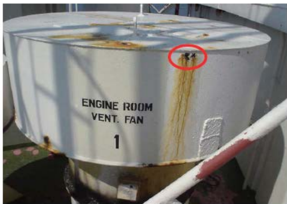
Corrosion holes in the casing of ventilator
