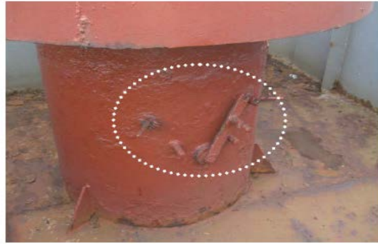
No marking of "Open-Shut"
