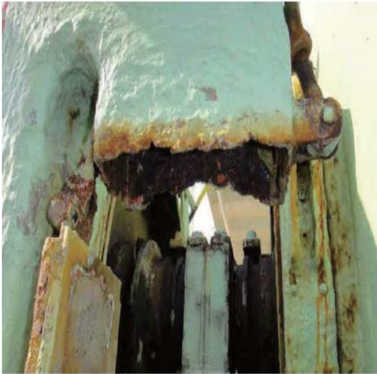
Wasted gooseneck ventilator
