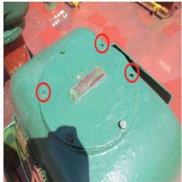
Missing bolts of air pipe head
