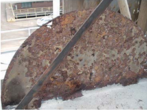
Wastage/Corrosion holes in fire damper flap
