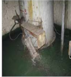
Hydraulic operated closing device not in good working condition
