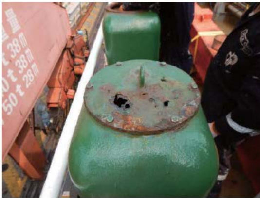
Corrosion holes in air pipe head
